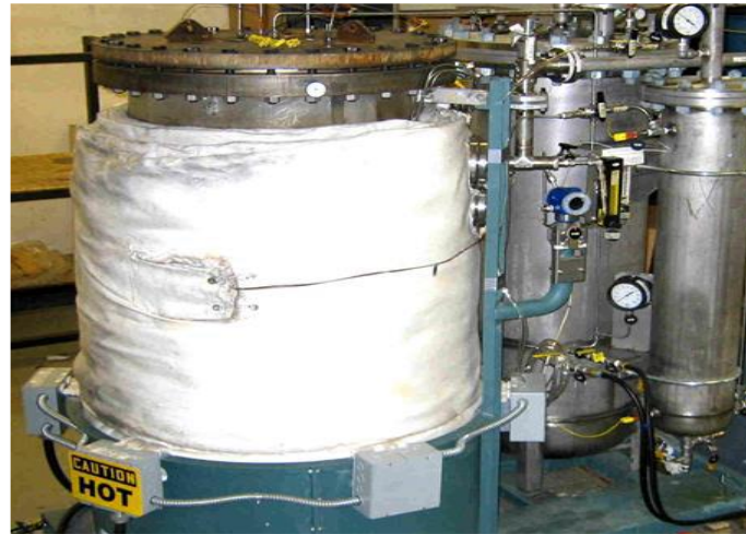
In Drum Pyrolysis
